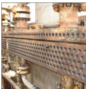
FinFan cooler before a maintenance
